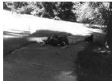
Sidewalks raised by roots create hazards.
